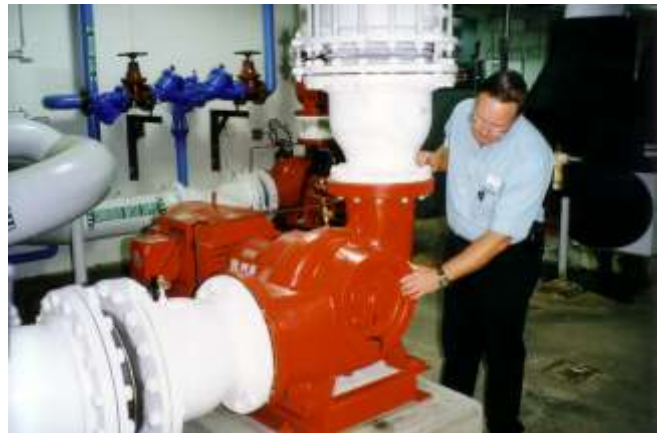
Bell & Gossit pump moves 3,200 gallons of chilled water per minute to the live animal attractions.
