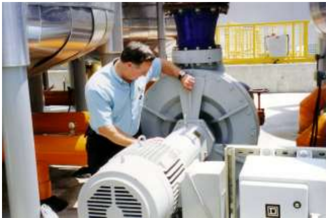
Fybroc carbon filter pump. It pumps 6,000 gallons per minute of salt water. It is protected with LE's 6413 Low Tox Turbine Oil.
