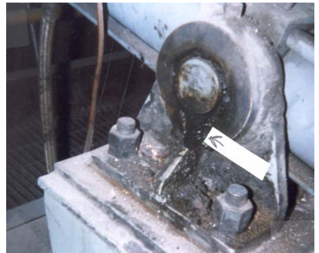
Grease dripping out of pin & bushing before using LE's 4701
